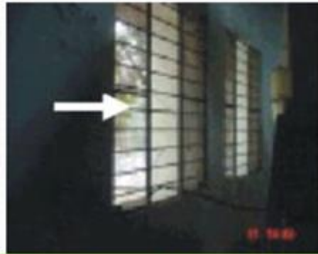
Broken glass of the window
