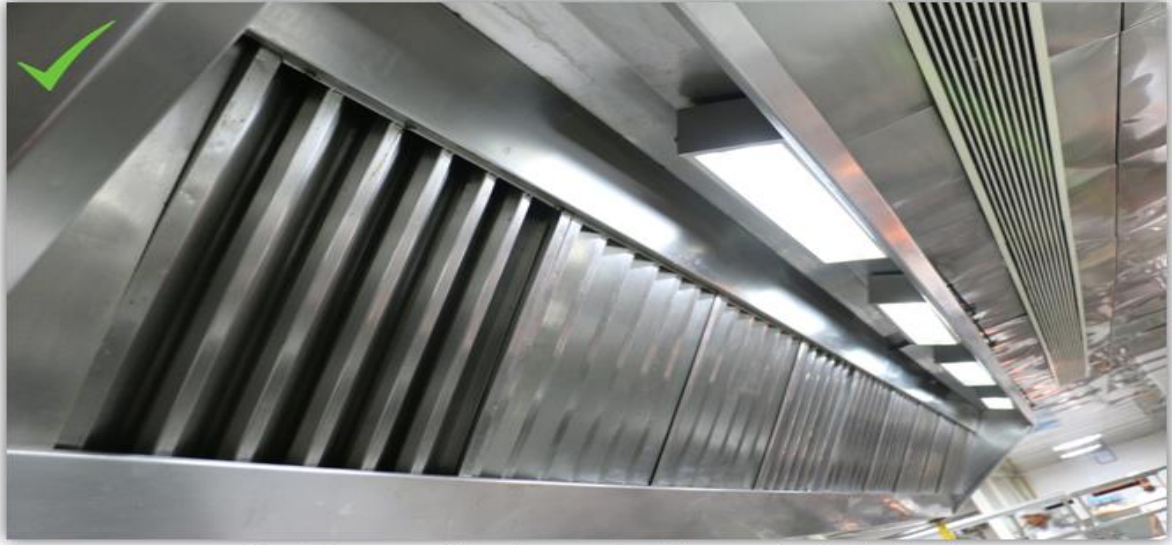
Food Preparation Areas shall have a installed chimney
