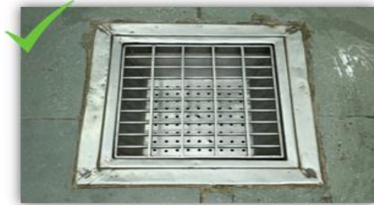
Drains should be covered to prevent insects and rodents
