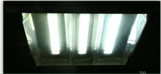
Lights shall be covered
