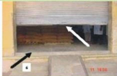
Gap in between shutter & floor
