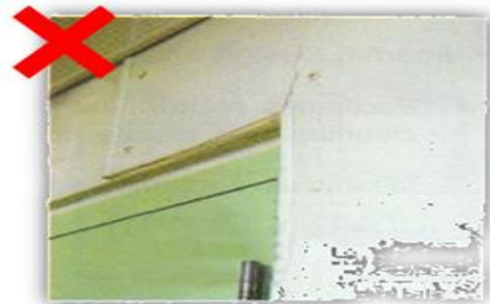
Cracks allow bacteria and molds to accumulate
