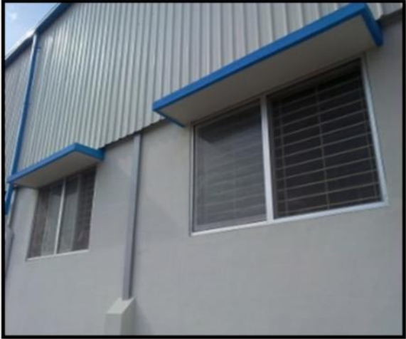
Netlons and mesh in windows to avoid pest entry
