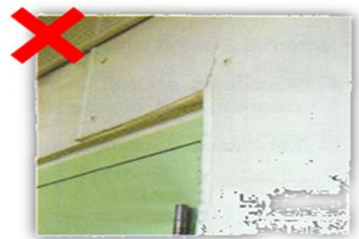
Cracks allow bacteria and molds to accumulate
