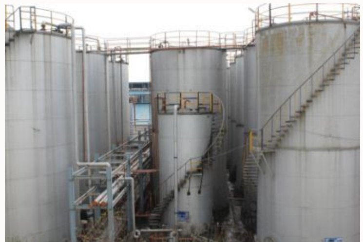
Dedicated Storage Tanks
