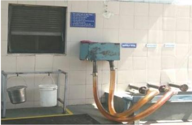
Covered Flexible Hose Opening to avoid Product Contamination
