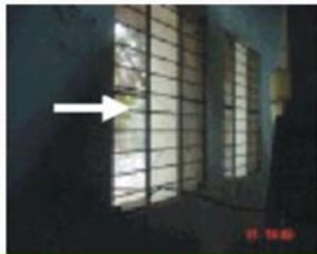
Broken glass of the window
