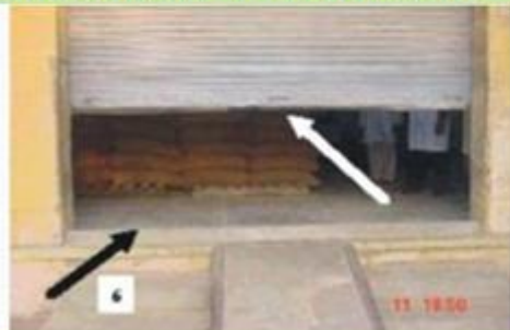
Gap in between shutter & floor
